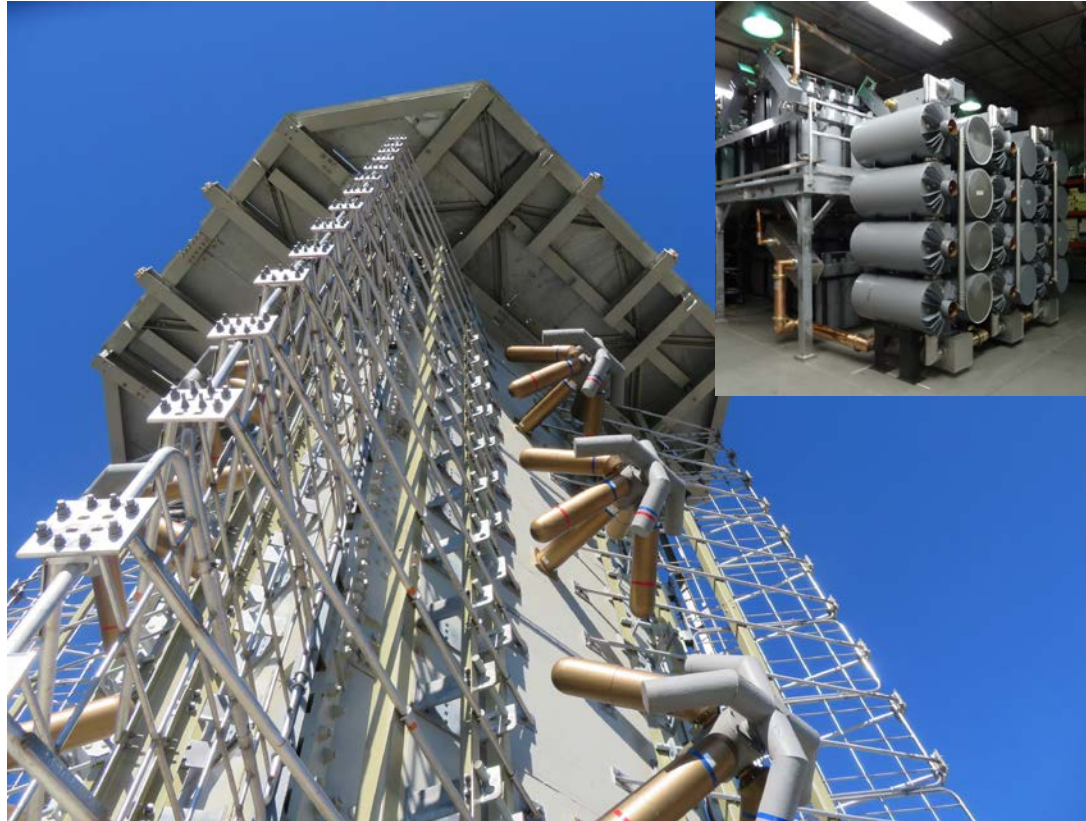
Empire State Building 19 FM Station Auxiliary FM Antenna and Channel Combiner System
